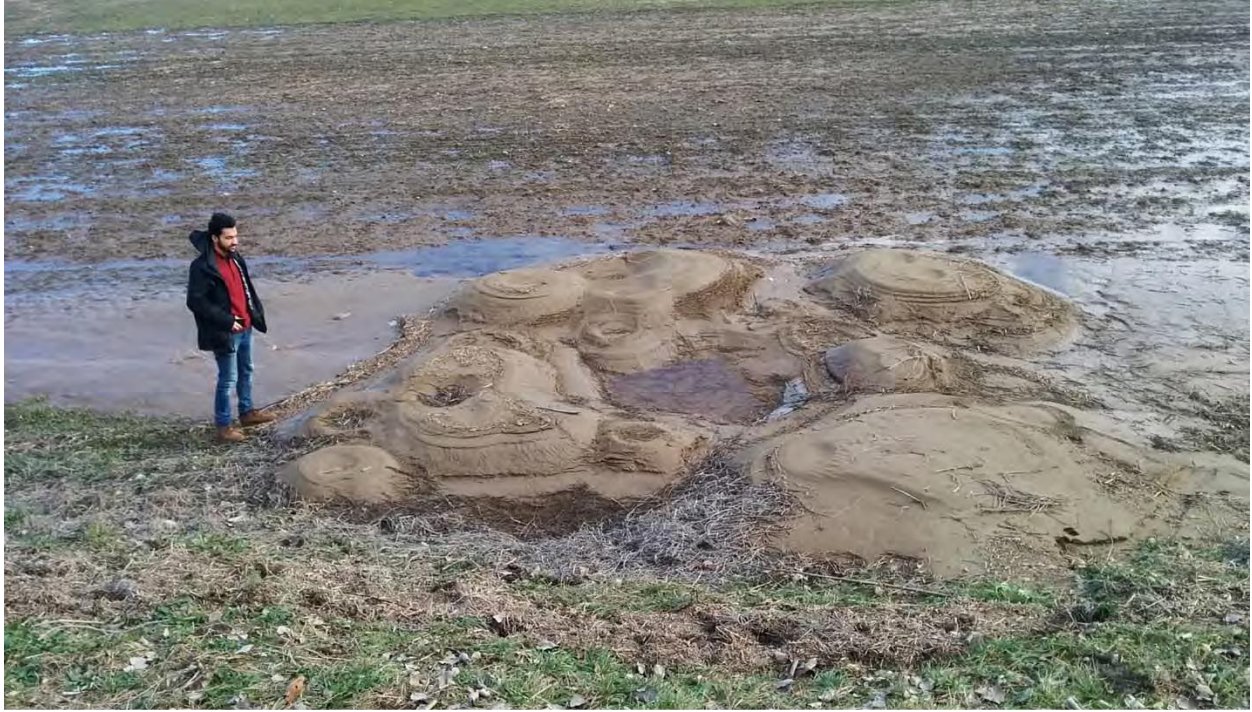
Figure 7 - Large sand boil network at levee toe near Olive Branch, IL (Rutherford et al., 2016)
