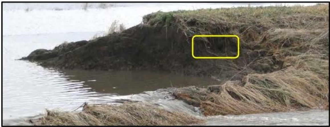
Figure 6 – View looking at exposed western edge of breach in a levee revealing the presence of animal burrows within the levee (Rutherford et al., 2016)
